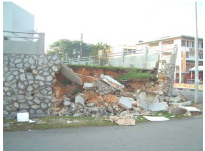
Figure 13: Collapsed Rubble Wall
