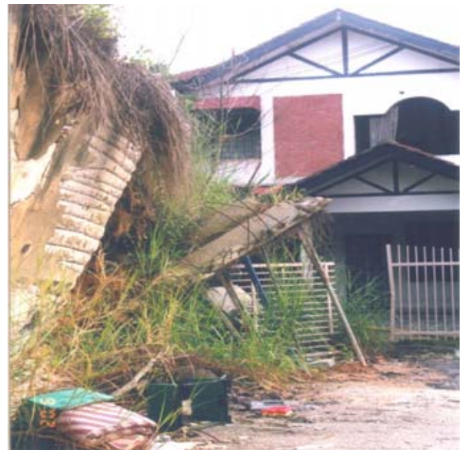
Figure 14: Failed RC Wall
