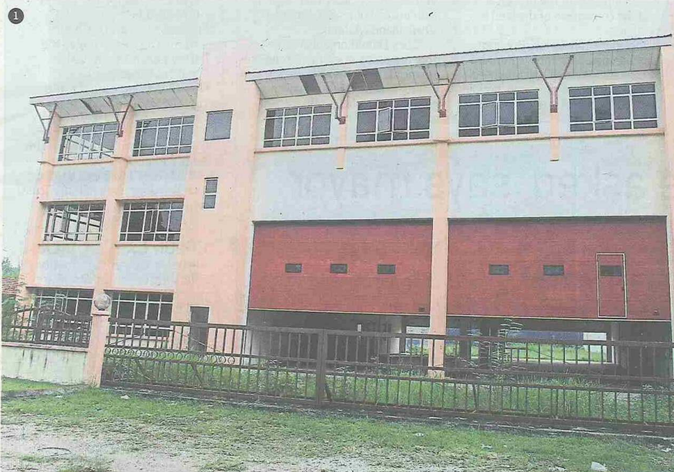
1 The Fire and Rescue Department In Jelatek which was 90% complete, had stalled because the developer faced financial difficulties.
